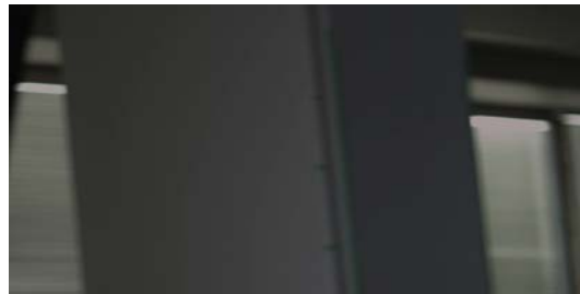
Figure 6. On frame 5, the wall appears to lean towards the left.
