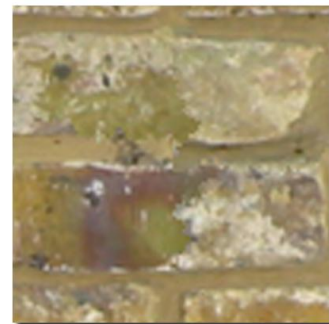
Figure 37.2 Furnace tiling with a vertical jagged line between tiles.
