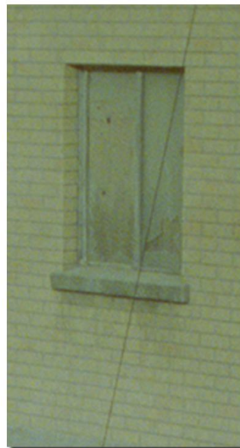
Figure 35.1 Cropped image of a wire across a brick wall.
